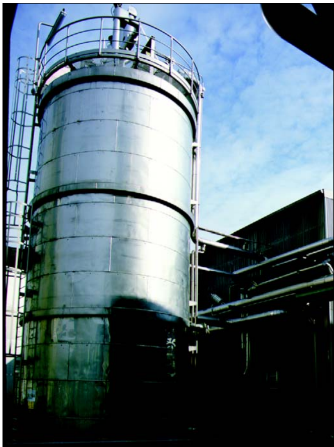
Figure 4. The tanks for intermediate storage of the purified water are filled with ozonized water.
