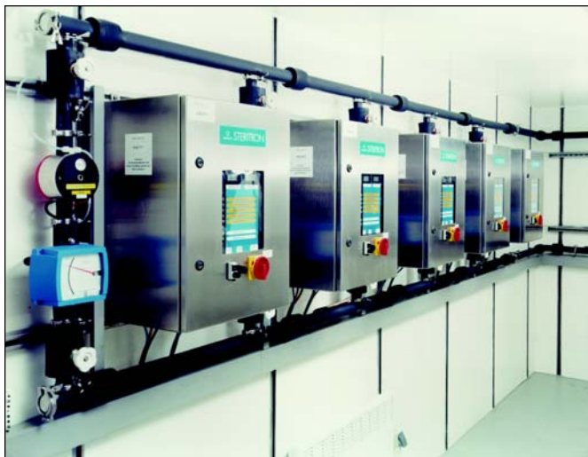
Figure 6. The ozone generators, some installed centrally, some at the consumer locations, add ozone to the water to achieve a concentration of 20 ppb.
