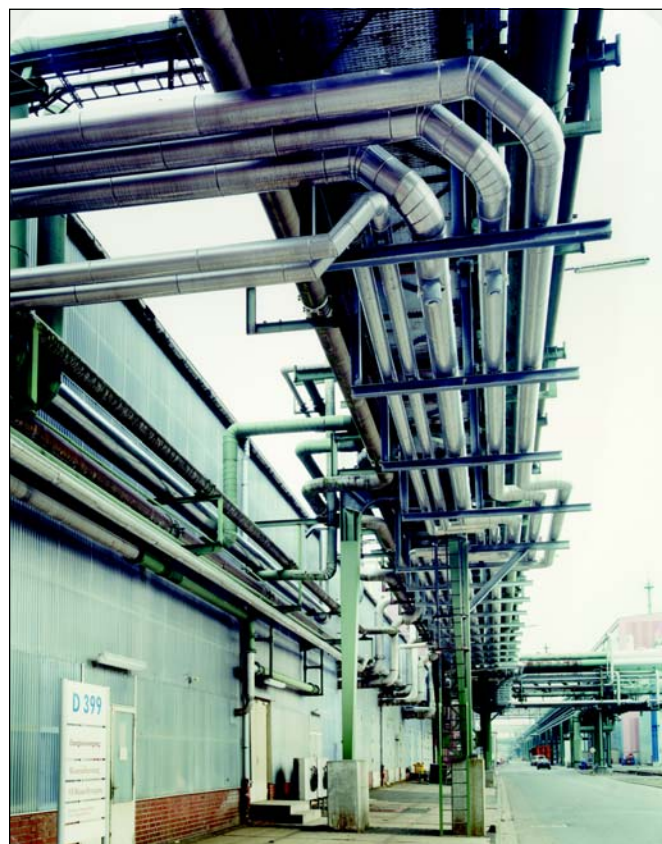
Figure 5. The pipes which carry the purified water to the 20 consumers extend over 14 kilometers.
